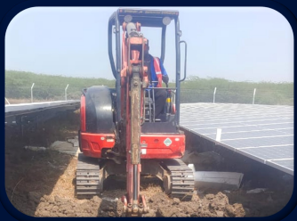
21MW Solar Power plant Sunsource Energy / ARKEN Solutions MCS works, Tamilnadu, 2024
