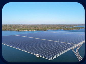
140MW Floating Solar Power plant AMP Energy / ARKEN Solutions MCS works, Madhya Pradesh, 2024
