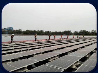
10MW Floating Solar Power plant UCL / Goodwill Engineers BOS works, Jharkhand , 2023
