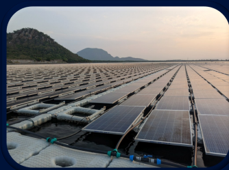
5MW Floating Solar Power plant Larsen & Turbo MCS works, Andhra Pradesh, 2023
