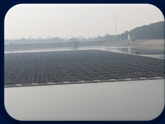
9.4MW Floating Solar Power plant Aditya Birla / ARKEN Solutions MCS works, Madhya Pradesh, 2024
